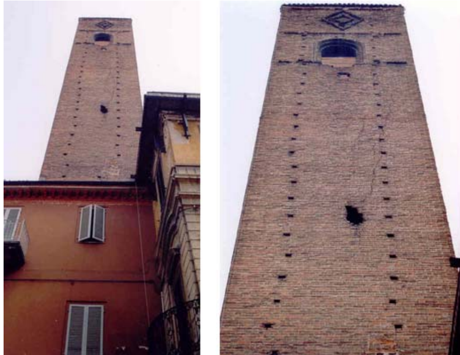
Astesiano tower, crack pattern of the sud view
