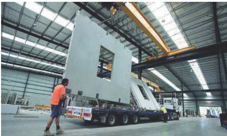
Fig. 1.23 Precast concrete panels are loaded on the trailer to be delivered (Url 13)
