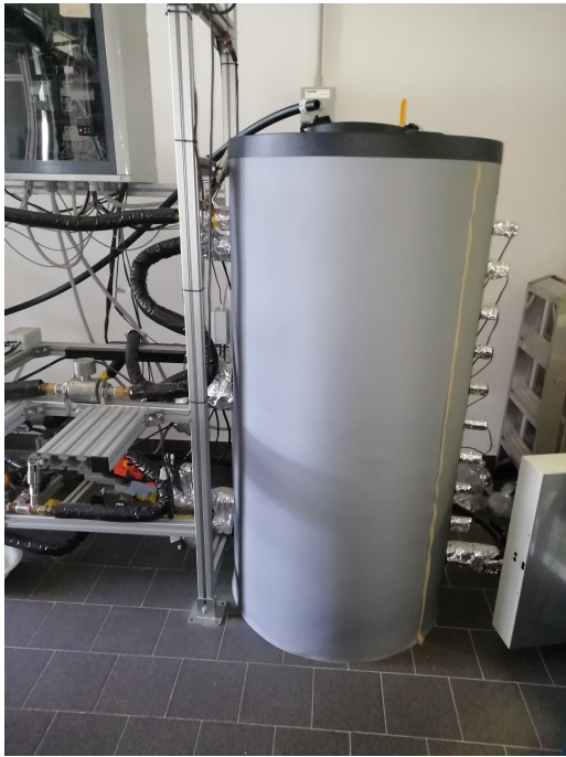
(a) Water tank
