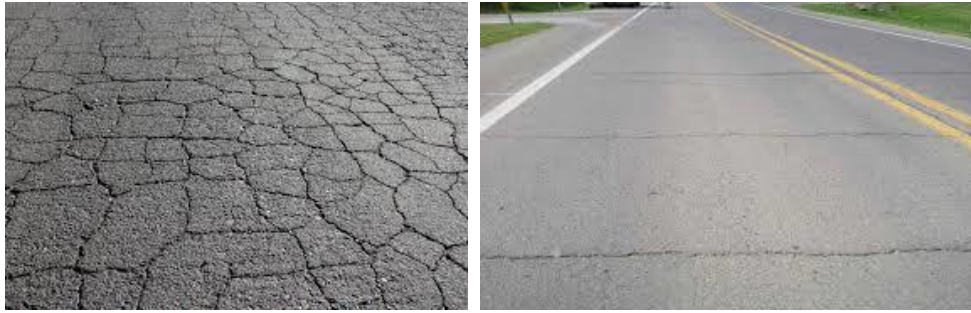
Figura 2.6: Alligator cracking e thermal cracking
