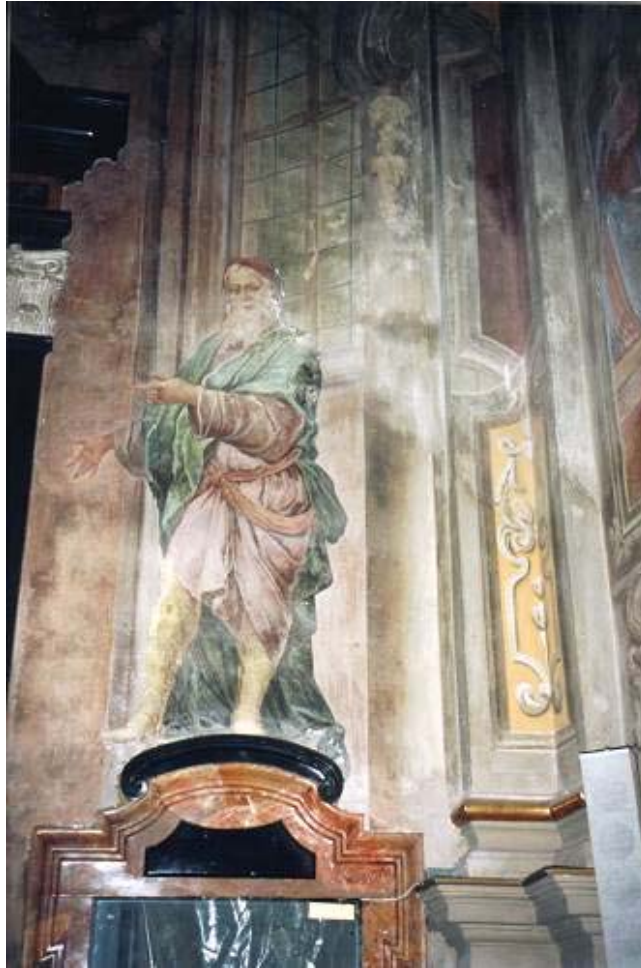
Deteriorated fresco in the church
