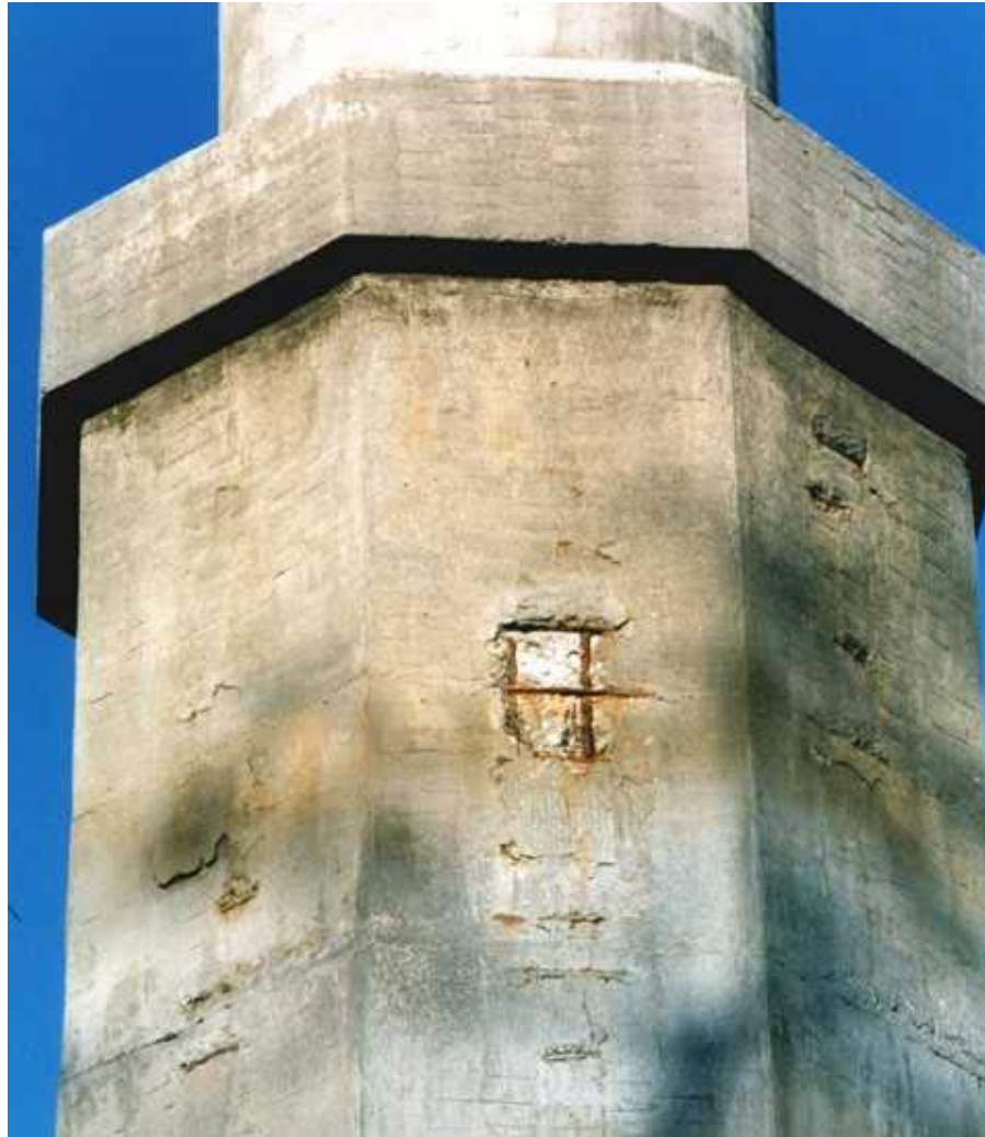
Concrete cortical disjunction
