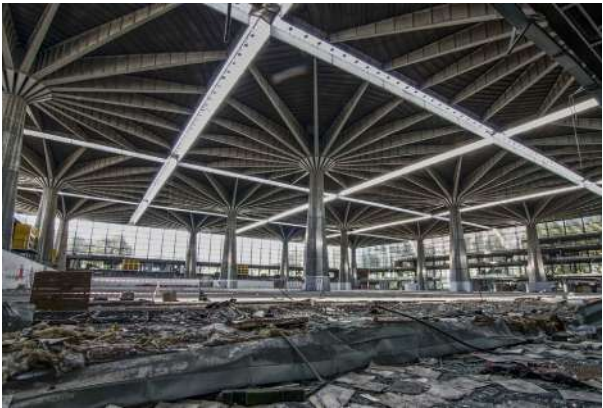
Figure 1.16: Interior after fire devastation.
