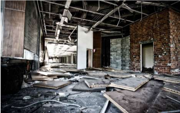
Figure 1.14: Interior after fire devastation.
