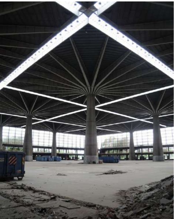
Figure 2.9: Palazzo Nervi after fire devastation and attempted renovation.
