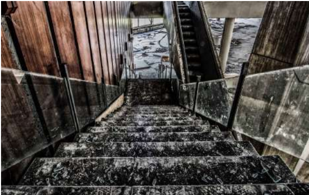
Figure 1.19: Interior after fire devastation.
