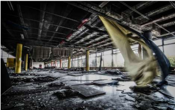
Figure 1.15: Interior after fire devastation.
