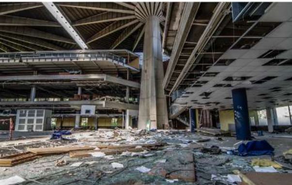
Figure 1.18: Interior after fire devastation.
