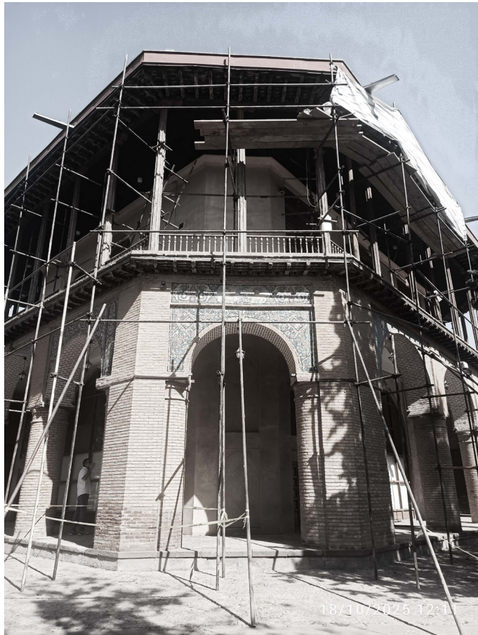
Figure.26 Chehelsotun Palace, Qazvin,Iran. Under maintenance to fix some damages accrued due to rain and snow.
