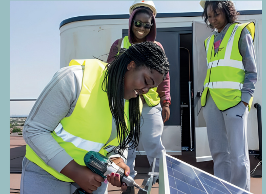
Figure 4. Community-owned solar energy project in London. (Repowering London, 2018)
