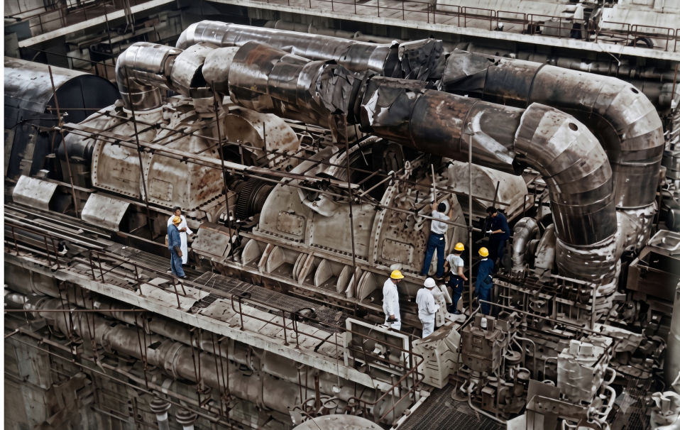
Figure 2.2: Aftermath of a catastrophic rotor/turbine failure caused by an undetected shaft or disc crack, illustrating the consequence of failing to identify crack growth before it reaches a critical size.
