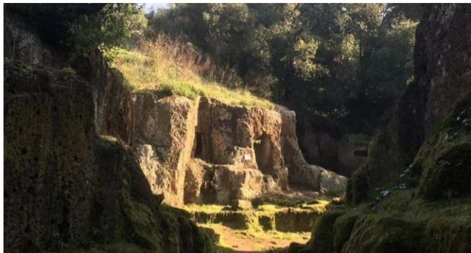
Figure 26. Vegetation interacting with rock-cut funerary architecture in the Cerveteri territory. The presence of moss, root systems and microclimatic shade illustrates the biological colonisation processes that affect the conservation of porous volcanic stone surfaces.
