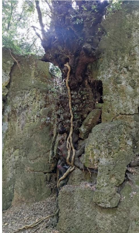
Figure 34. Vegetation growth and root penetration within the tuff rock of the Banditaccia necropolis, illustrating the impact of biological colonisation, moisture infiltration and long-term weathering processes on the structural integrity and preservation of tomb features.
