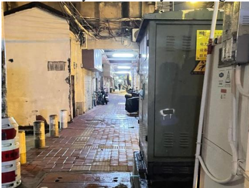
Electrical Installations and Overhead Wiring
