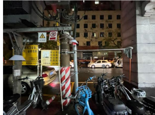
Electrical Facilities, Parking
