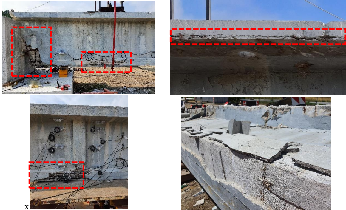
Figure 2.5. Main types of degradation observed on the beam.
