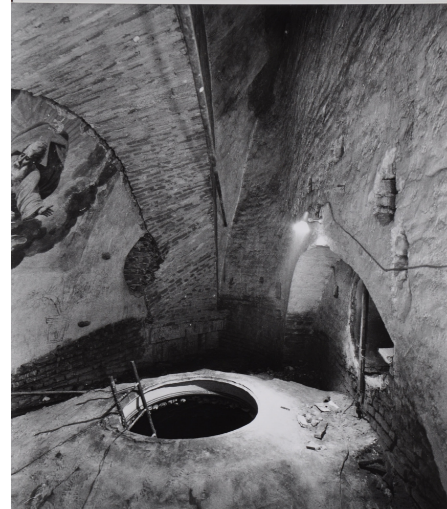
Figure 51 – The space between the star-shaped vault and the intrados of the squinch. From Franco Rosso, Guarino Guarini , 2006. Photograph by Giuseppe Dell'Aquila.
