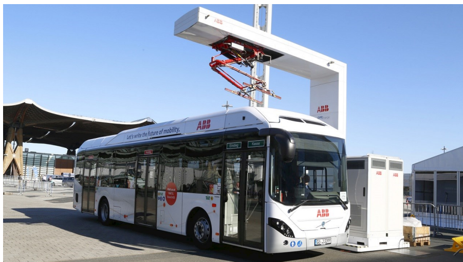
Figure 3.5: Pantograph Down - Real application
