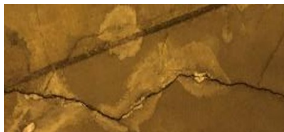
Figure 41 longitudinal cracks along the tunnel coating, aligned with the tunnel axis (MIMS, 2022)
