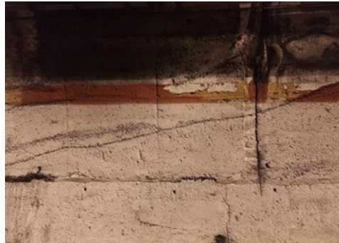
Figure 42 Diagonal Cracking (MIMS, 2022)
