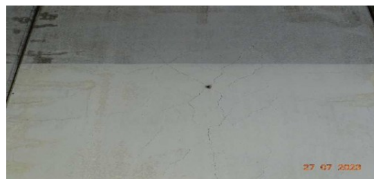
Figure 51 shrinkage cracks on a segment surface
