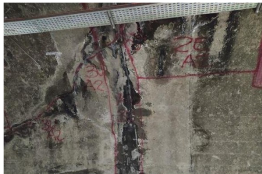
Figure 48 Deterioration of concrete joints. (MIMS,2022)
