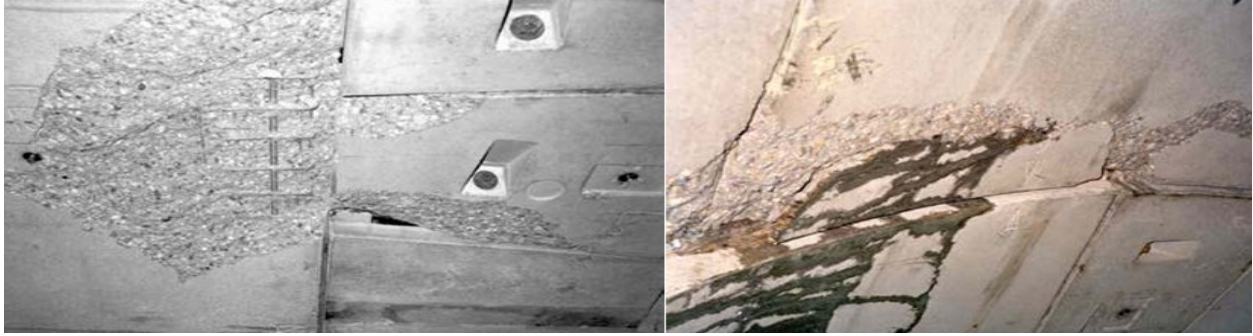
Figure 27 Splitting transversal cracks (SIG WG2, 2019)
