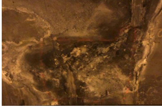
Figure 34 White coatings on surface of concrete (MIMS, 2022)
