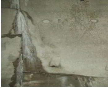
Figure 24 Water leakage from joints (SIG WG2, 2019)
