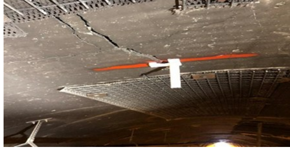
Figure 37 Visible cracking and material detachment on a tunnel ceiling caused by compressive stress (MIMS, 2022)
