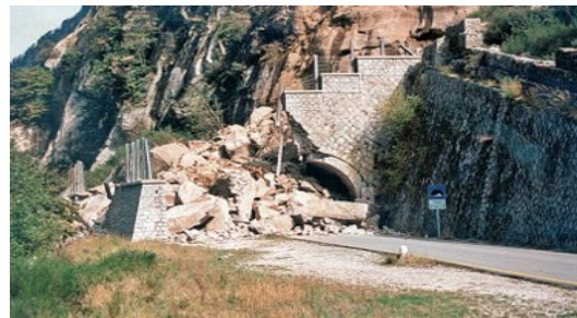
Figure 36 slope instability causing debris flow & structural damage on tunnel entrance (MIMS, 2022)
