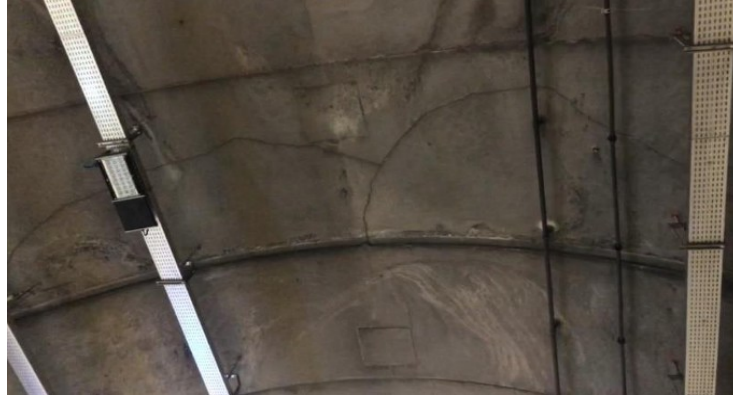
Figure 43 Curvilinear cracks observed in the tunnel lining (MIMS, 2022)
