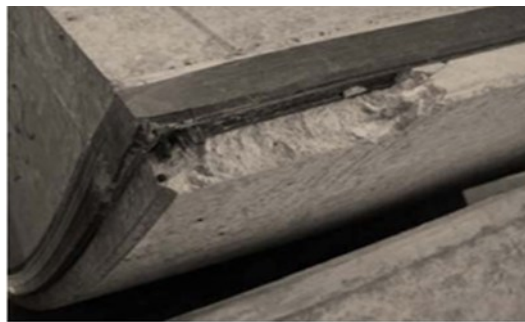
Figure 16 Example of corner breaking (SIG WG2, 2019)
