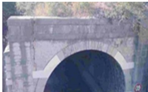
Figure 35 Deterioration of the entrance portals (MIMS, 2022)
