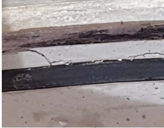
Figure 18 Chipping of edge during installation (SIG WG2, 2019)
