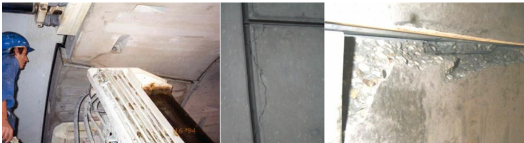
Figure 26 Segment cracks during erection (left) and ring erection (right) (SIG WG2, 2019)
