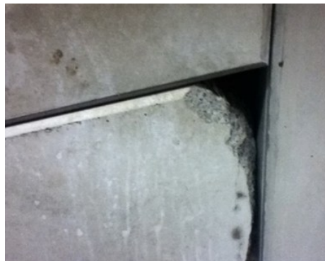
Figure 19 Chipping of corners during installation (SIG WG2, 2019)
