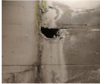
Figure 47 void formation behind the intrados of the tunnel lining. (MIMS,2022)
