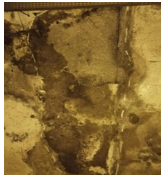
Figure 49 Surface Defects (MIMS,2022)
