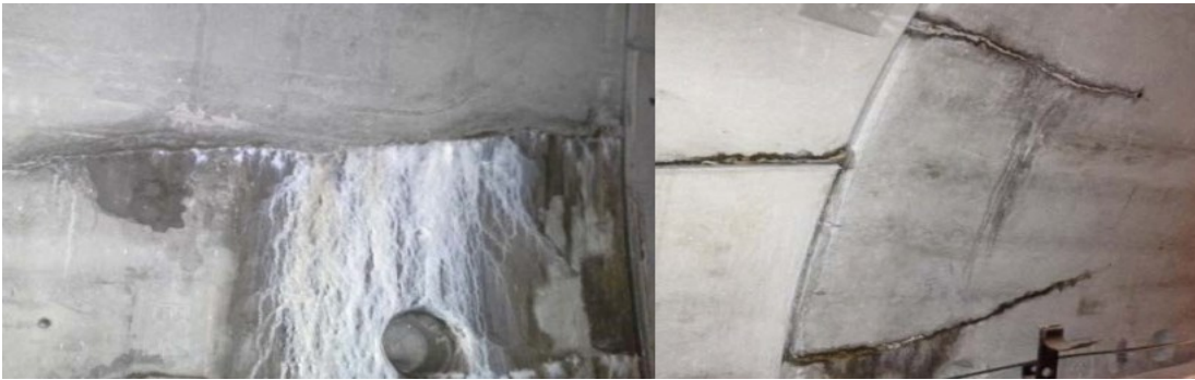
Figure 28 Longitudinal cracks along the tunnel and spalling cracks (SIG WG2, 2019)
