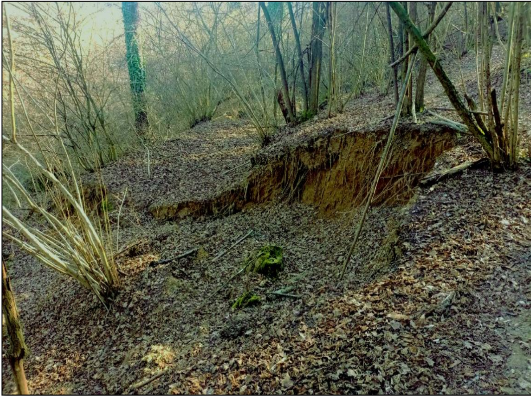
Photo 1: Existing Collapse at the side of the tunnel's entrance from the North
