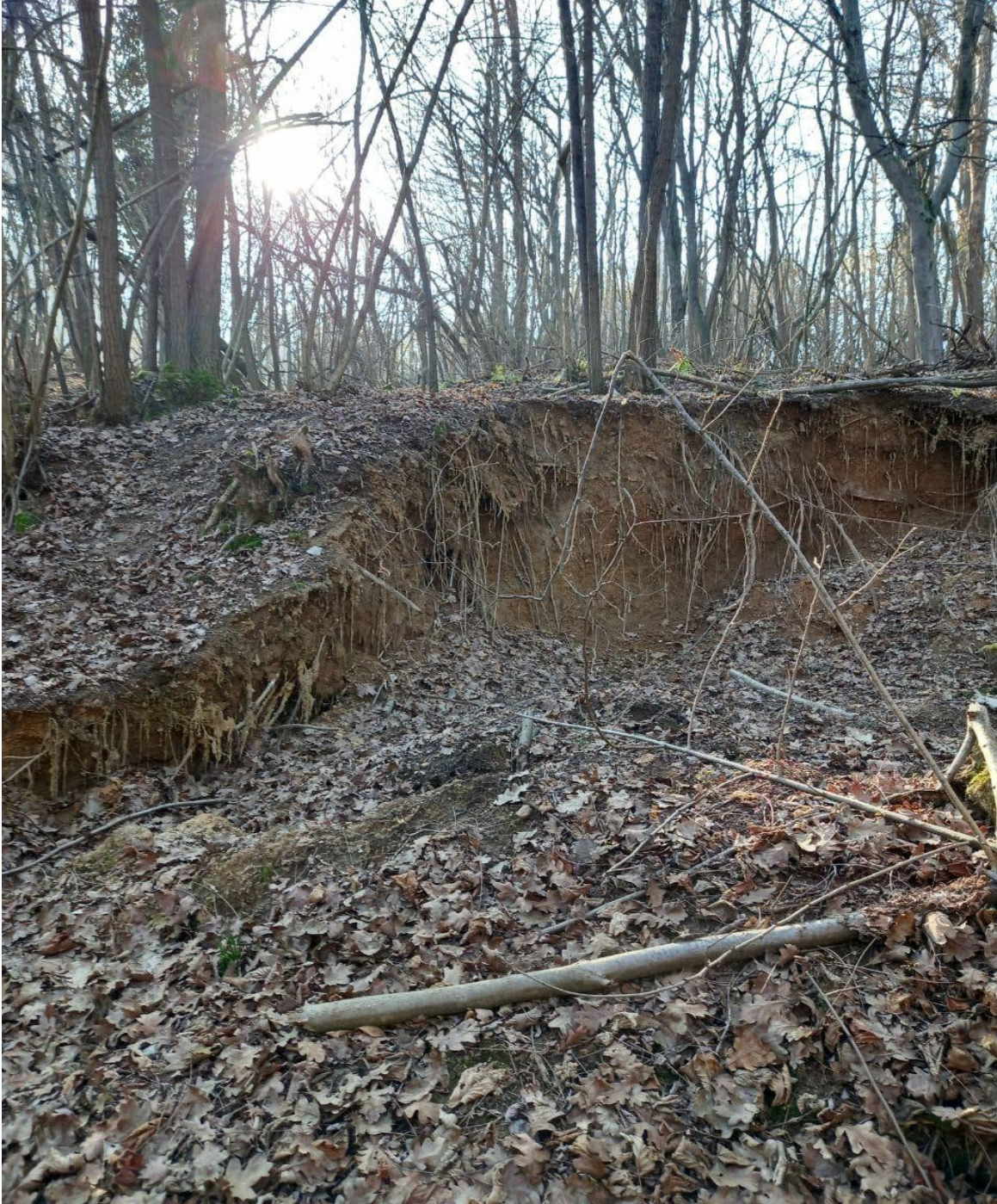
Photo 2: Existing Collapse at the side of the tunnel's entrance from the North
