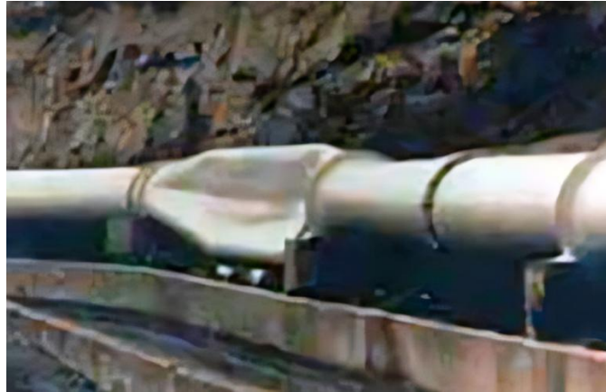
Figure 45: collapsed pipe due to water hammer (source: Harper Haines website )
