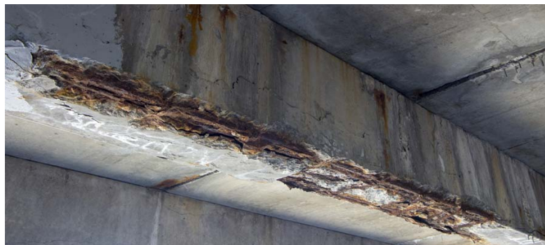
Figure 3.1. Concrete degradation in a bridge deck [20]
