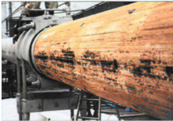
Figure 3.11. Corrosion on the side of a cable from the Innoshina Bridge [58]
