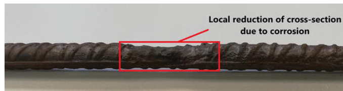
Figure 3.6. Pitting corrosion on a rebar [32]
