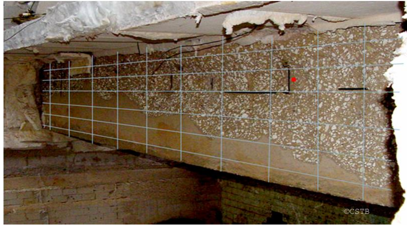
Figure 2-20[20]: Example of grid for spalling depth distribution analysis.
