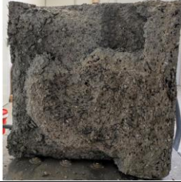
Face before and after fire
