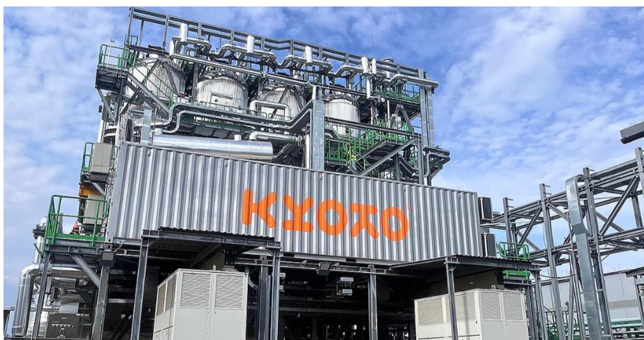
Figure 3 The largest industrial thermal energy storage system, at KALL Ingredients' corn processing facility in Tiszapüspöki, Hungary. From Kyoto Group website
