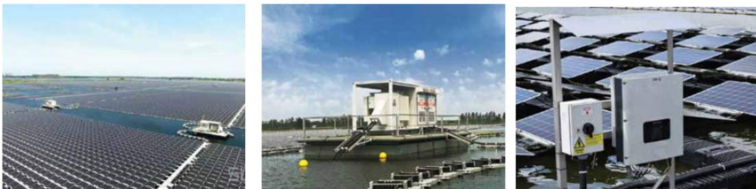
Figure 2.8: Floating solar farm equipped with a central inverter installed on a dedicated floating island and distributed string inverter mounted directly on the floating array (source [10])
