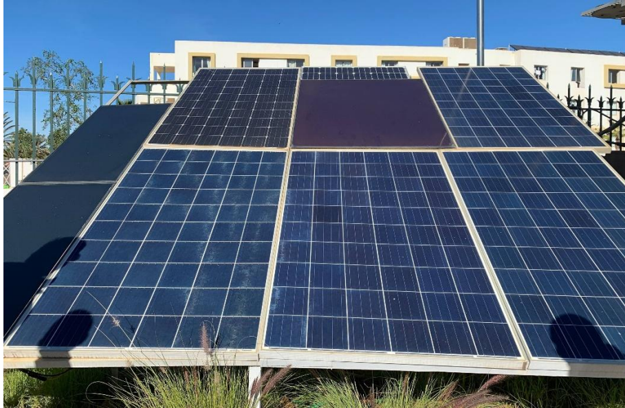
Figure 5.1 – Residential PV power plant of the International University of Rabat.
