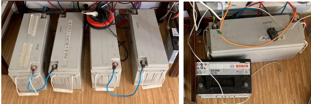
Figure 5.7 - Battery storage configuration of the UIR power plant.
