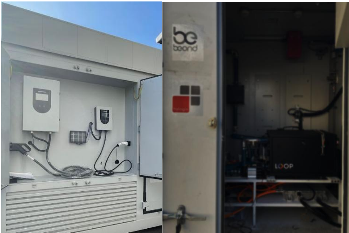
Figure 3 SIRIH2 charging station(left) and hydrogen power cell(right)
