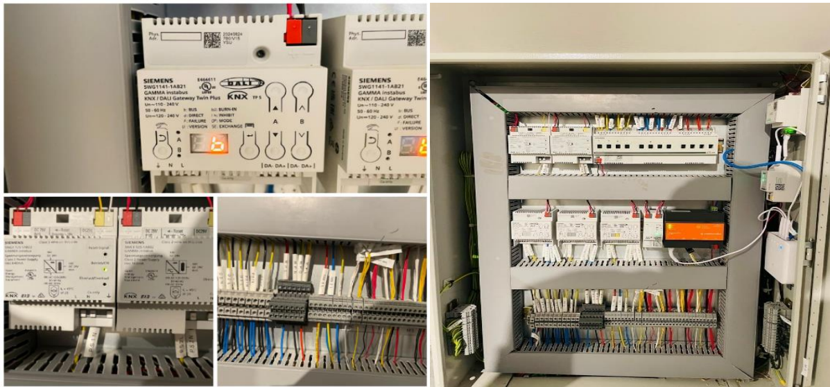
Figure 11 KNX Automation Panel Installation
