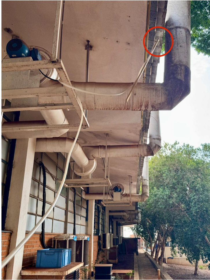
Figure 3.12: Outlet line through which the purified gases are released after passing through the scrubber. Credit: Author
