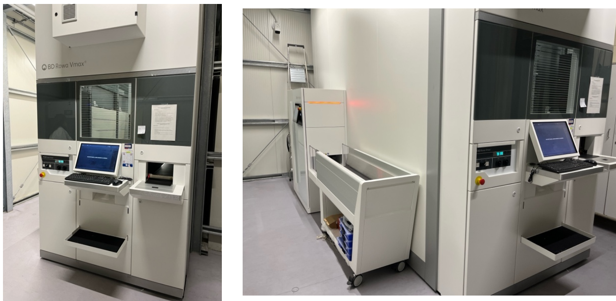
Figure 13: BD Rowa VMax located in Direct Distribution storage area
