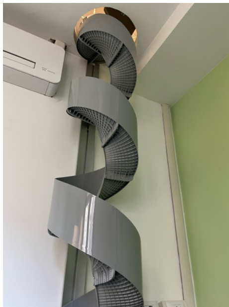
Figure 14: Spiral vertical delivery duct transporting medications from the BD Rowa VMax to the pharmacy dispensing offices
