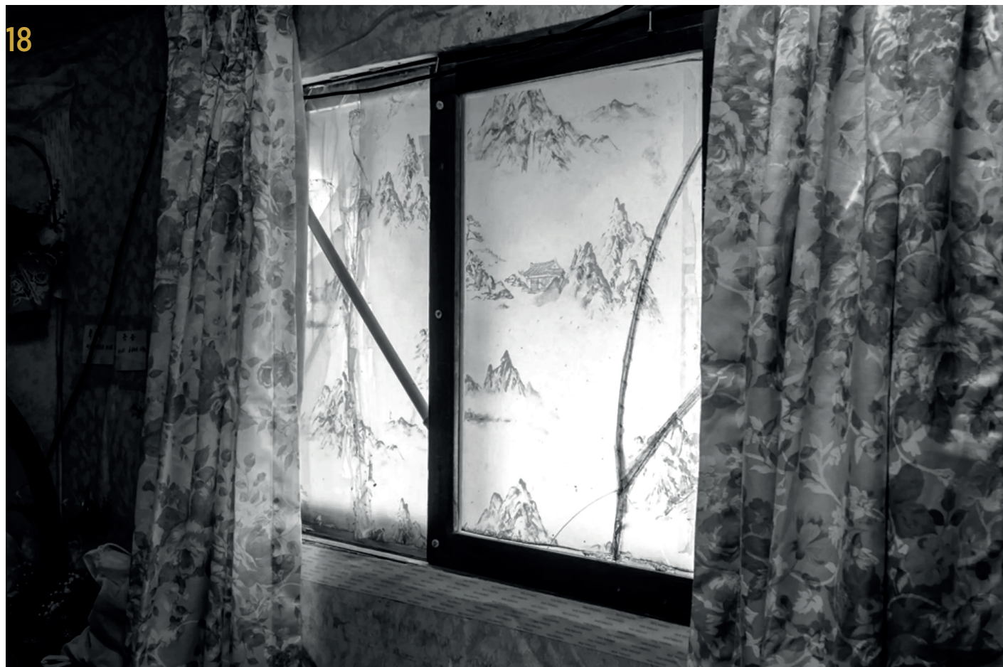
1.1.3 Window with deteriorated walls , Stachmann, R., 2023
