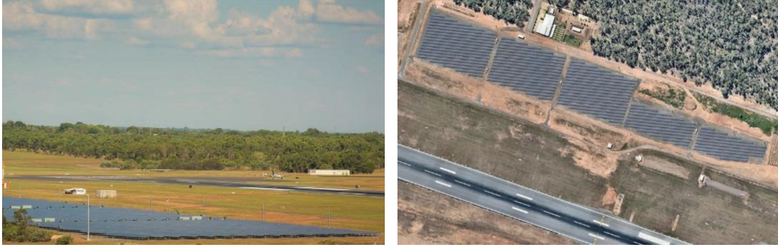
Figure 5.8: Solar panel installations at Darwin International Airport
