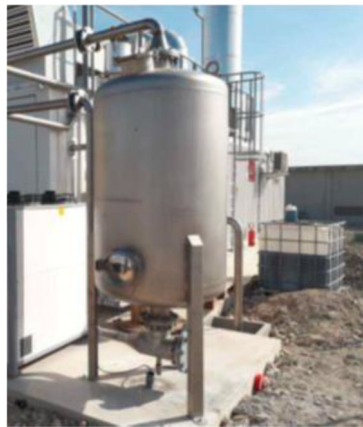
Figure 20 : Activated carbon filter
