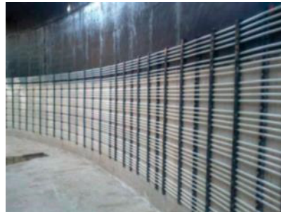
Figure 16 : Example of a coil placed on the walls for thermostating the digester
