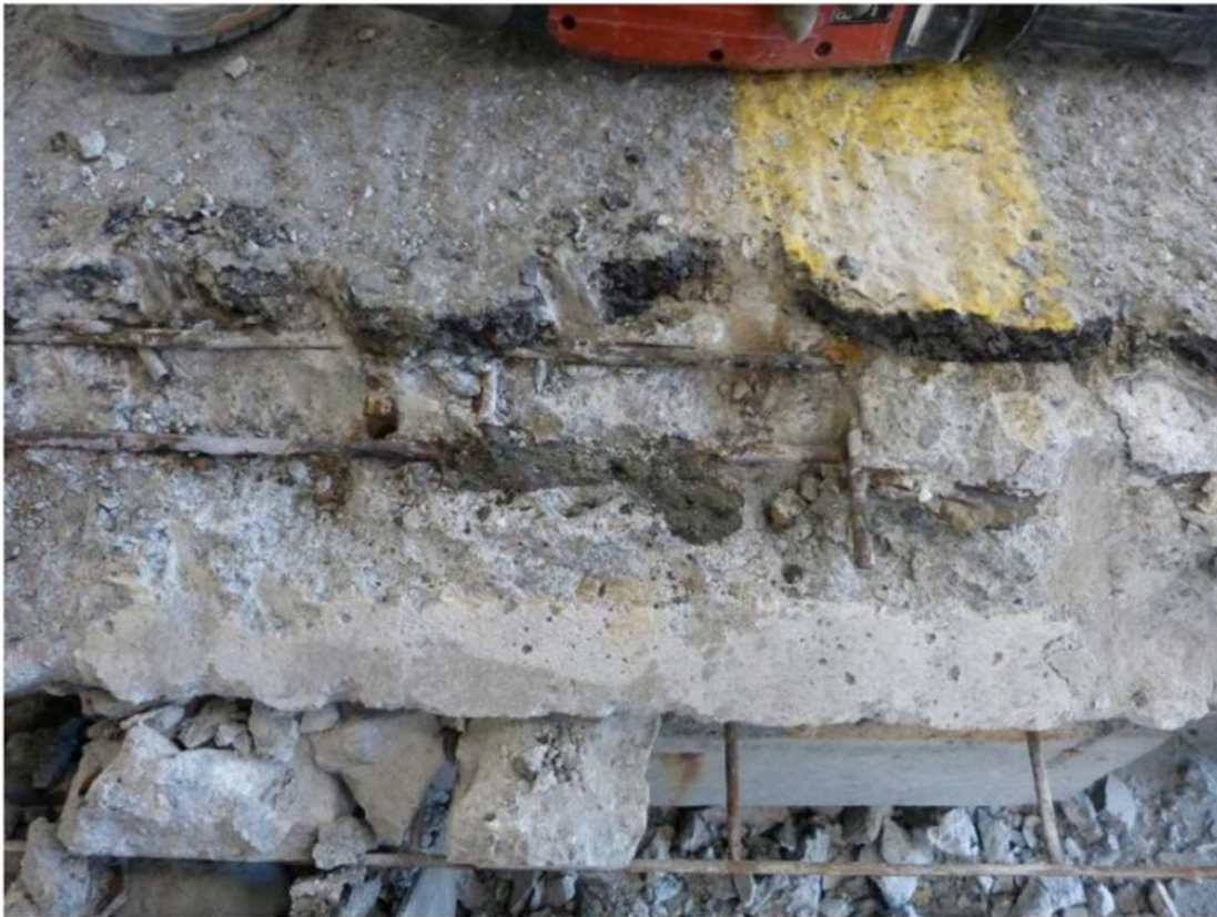
Figure 87: Degradation of reinforcement in cast-in-situ joint
