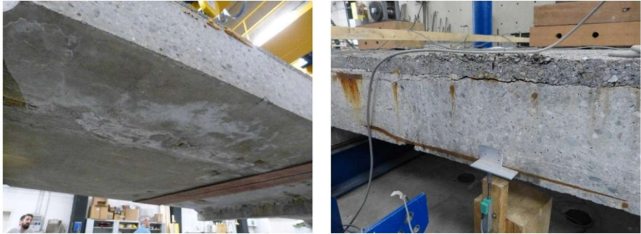
Figure 21: Left - saline efflorescences on span 1. Right: Crack pattern on span 3
