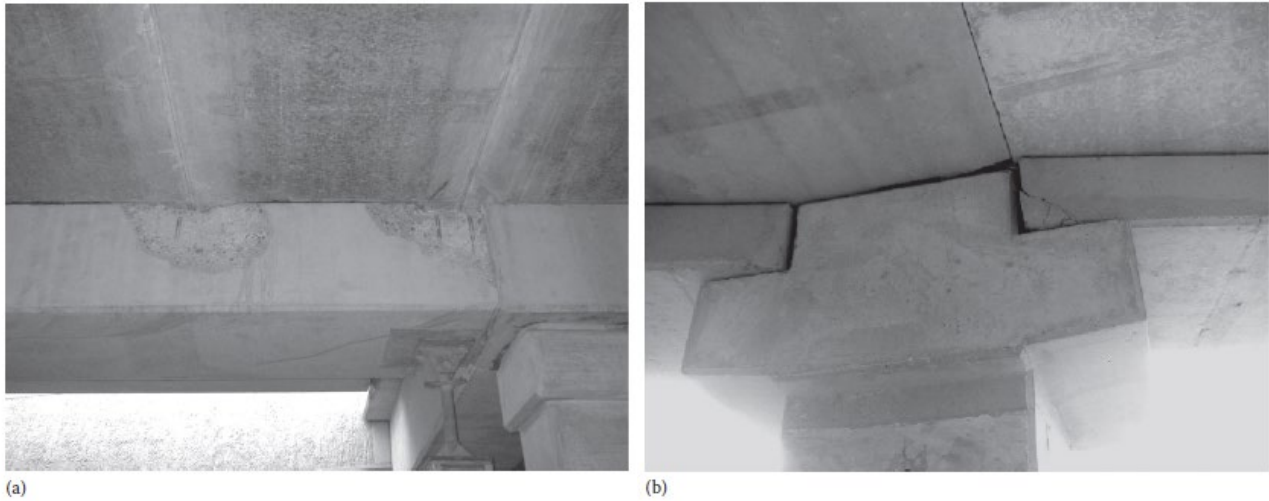
Figure 5 a) Spalling due to relative movement between slabs and beams. (b) Cracking due to spurious restraint at a beam-to-column corbel connection.
