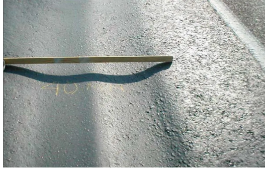
Figure 2.13: Rutting phenomenon in asphalt pavement.
