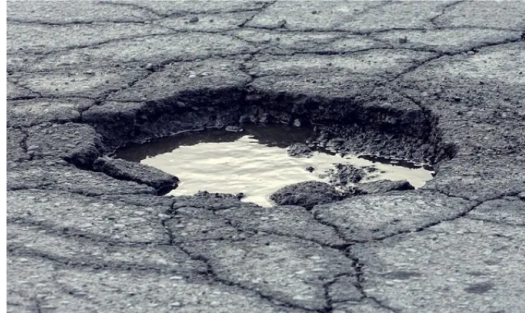
Figure 2.8: Potholes phenomenon in asphalt pavement.
