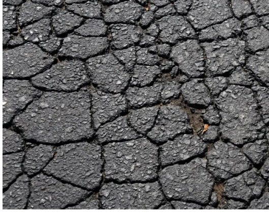
Figure 2.11: Fatigue cracking phenomenon in asphalt pavement.
