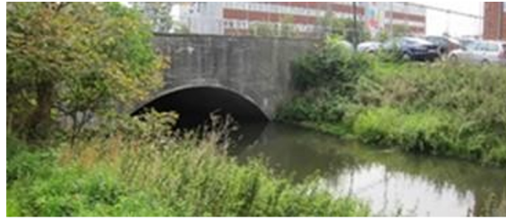
Figure A.4: Bridge over a river where the underpass must be widened to prevent bottlenecks during heavy rainfall [28].
