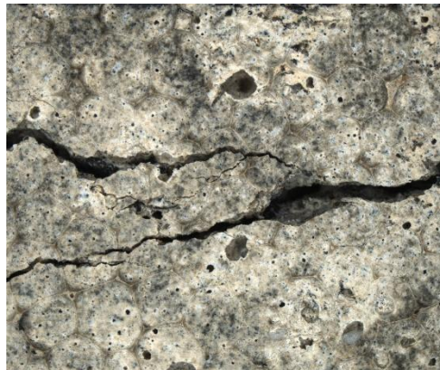
Figure 48 - Macro picture of a cracked matrix with pores
