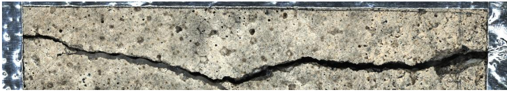
Figure 46 – Crack with visible fiber
