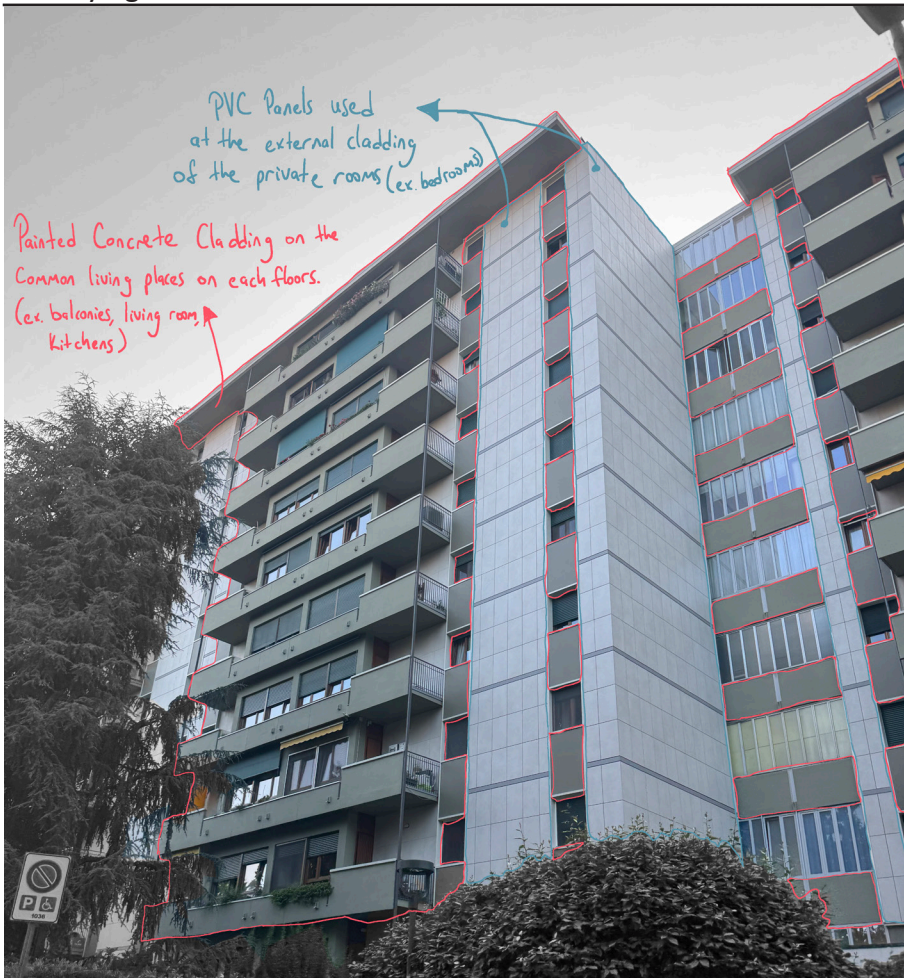
fig 120. Multi-story residential building with concrete structural elements and PVC panels as cladding, Intersection of Corso Unione Sovietica and Corso Eusebio Giambone 10134 Turin, Photo by the author, June 11 2025.
