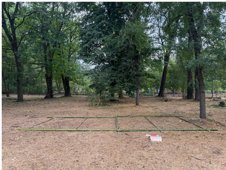
fig 356. One side of the structure is attached to the beam and other side is ready to be risen for the last pegs to be inserted at the end of the second workshop day, Photo by the author, July 23 2025.
