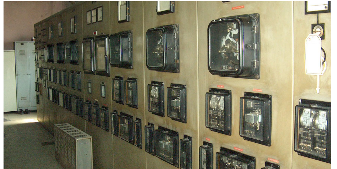
Fig 114: First Floor, Control Room
