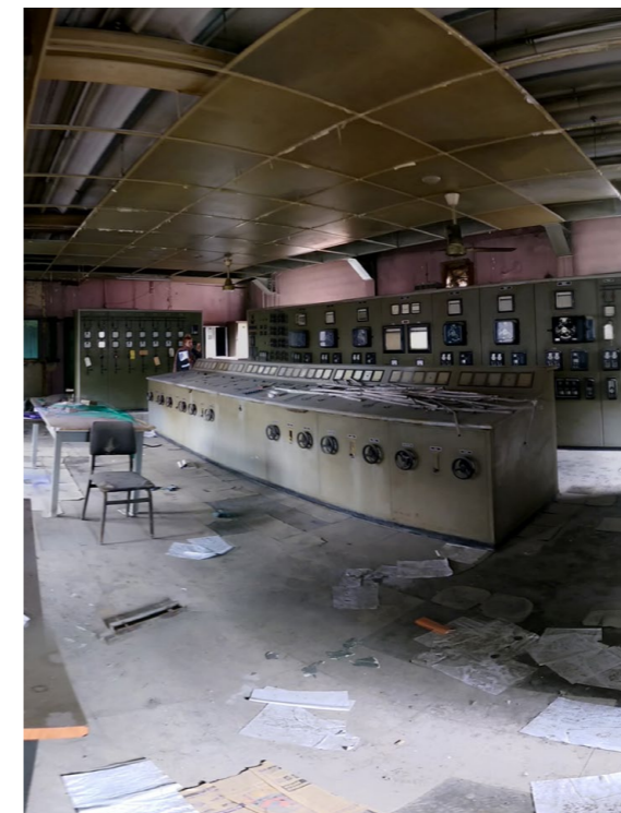
Fig 117: First Floor, Control Room
