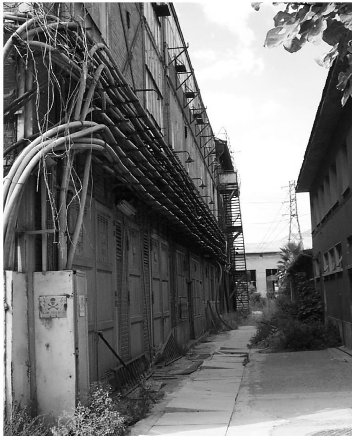
Fig 90: East Wall- Cable Distribution
