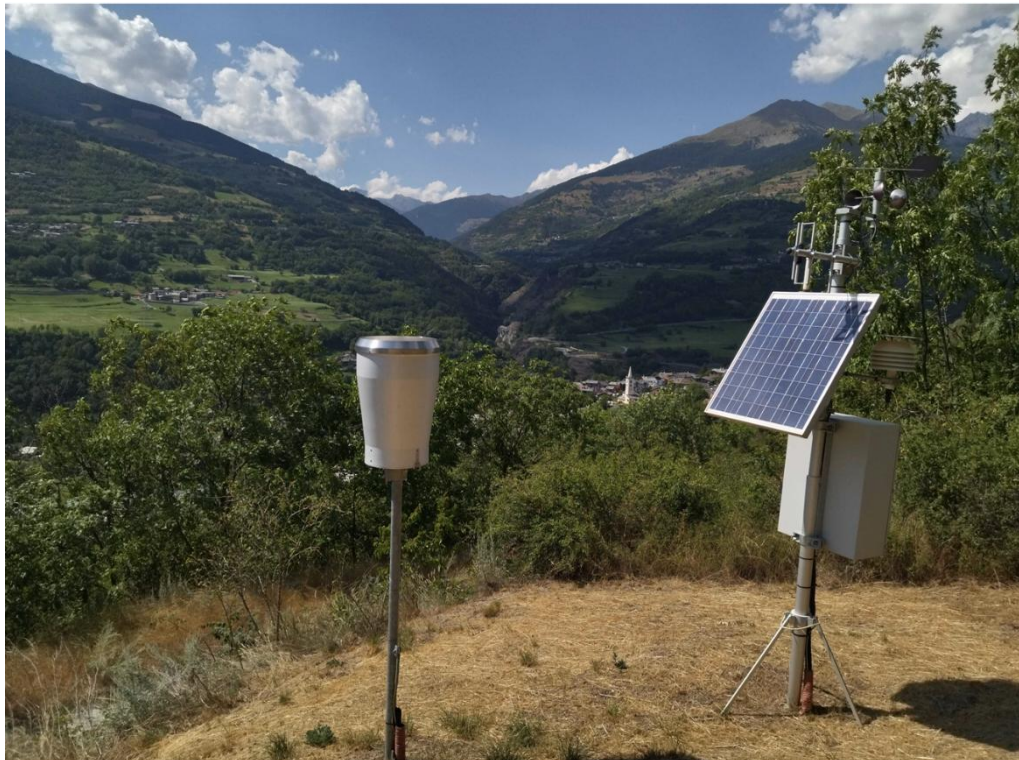
Figure 12 - Weather station of Roisan-Preyl equipped with a rain gauge for precipitation monitoring (on the left).
