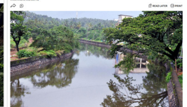
FOR A NEW LEASE OF LIFE: Strengthening of sidewalls to protect against encroachment forms part of the project to revive the Canoly canal. Photo: S. Ramesh Kumar
