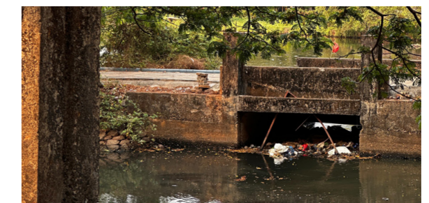
Figure 66 Waste water inlet between the canal into the wetlands (Source: Image by Authors)
