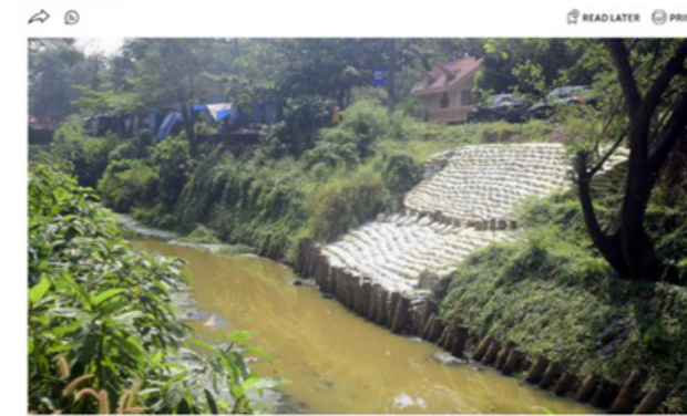
The protective walls of the Conolly canal being reconstructed at Karaparamba in Kozhikode.
