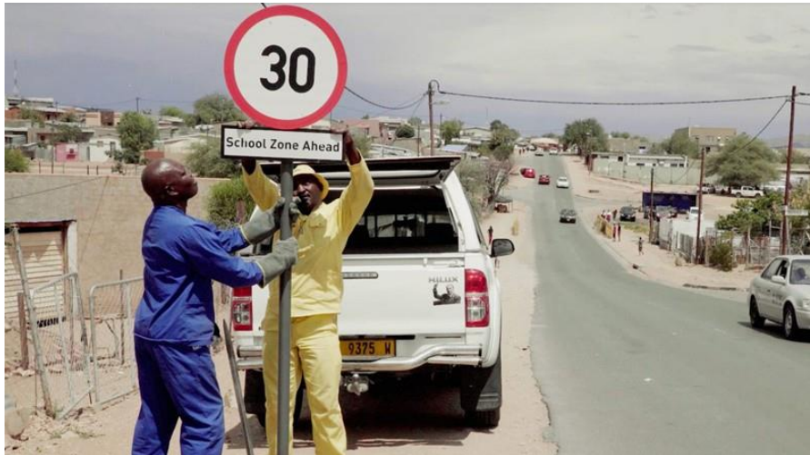
Figure 10: Installation of 30 K/h speed limit sign for school zones in Lusaka City Source: Child Health & Mobility.
