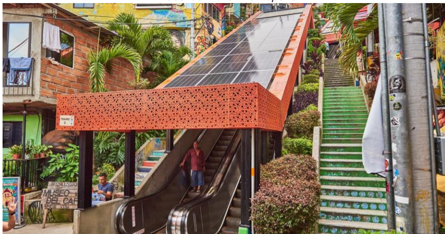
Figure 17: Escalator in Medellín now use solar panels as their energy source. Source: Telemédellin.tv
