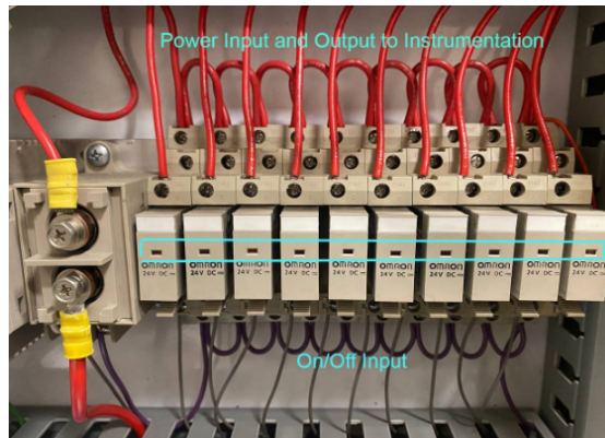
Figure 4.15: Relay box in the DAQ. The figure also shows the input and output cable arrangement
