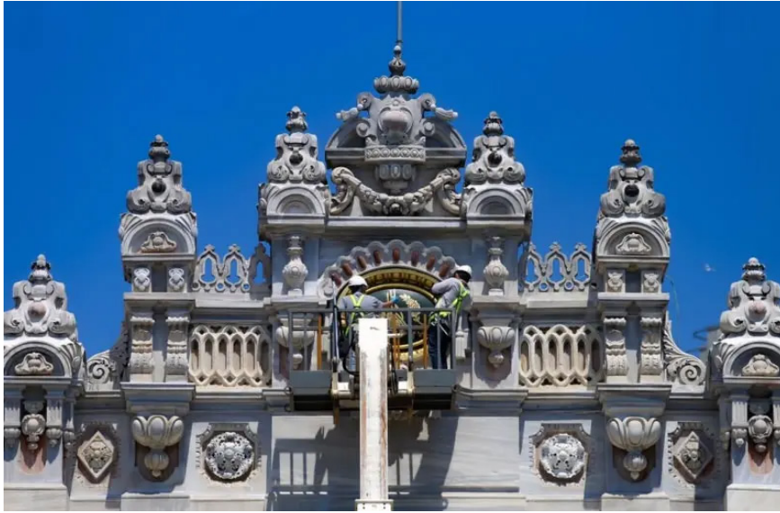
Picture of restoration work on the Gate of the Sultan in 2020, Dolmabahce Palace, Istanbul, Turkey ( https://www.haber7.com/seyahat )
