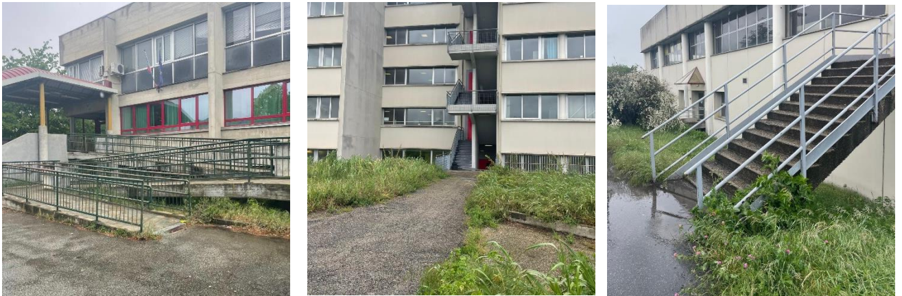
Figure 26 Conducted site inspections and updated models in Revit based on inspection results.
