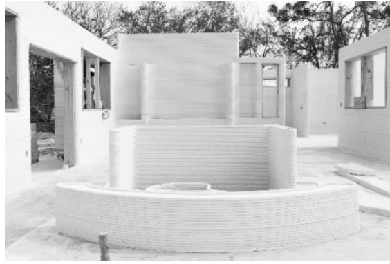
Image 4 Apis Cor's 3D-printed concrete walls for a residential house in Melbourne, FL. Soucre: (Apis Cor, a Manufacturer of Construction 3D Printing Robots, Announces Strategic Investment by D.R. Horton, 2024).
