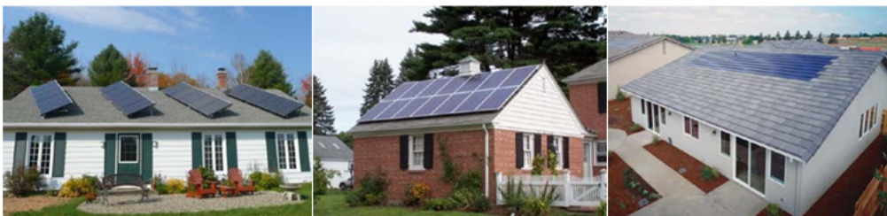
Least integrated (Open rack-mounted PV)
