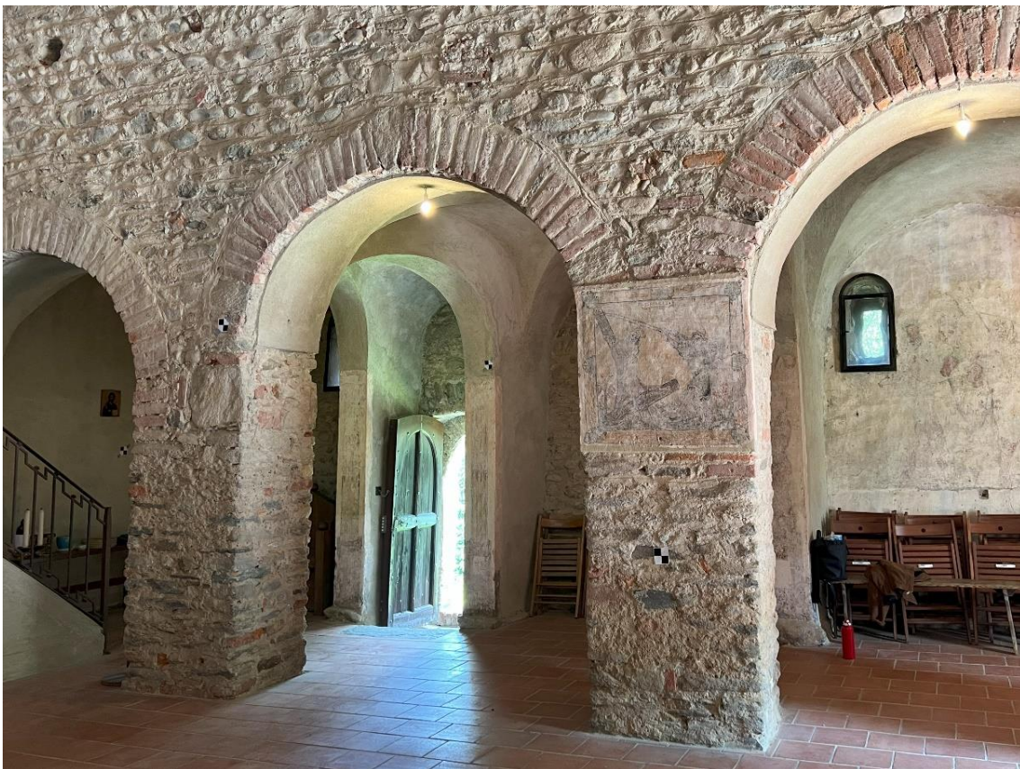
Image 4 - Rectangular columns and semicircular arches in the right nave of Santo Stefano church.
