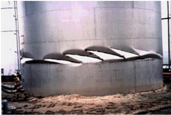
Figure 1-7: Diamond-Shaped Buckling (Courtesy of N R I of Fire and Disaster, Japan)
