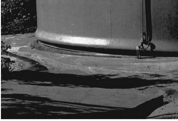
Figure 1-11: Elephant's foot buckling of the lower of the tank [11]
