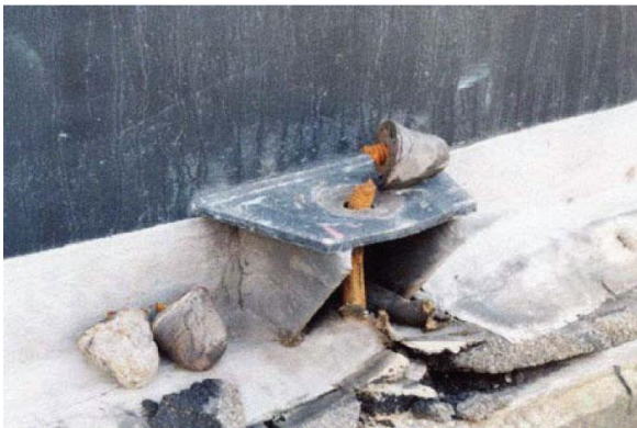
Figure 1-16: anchorage failure of a tank during Hanshin-Awaji earthquake [26]
