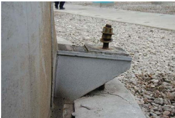
Figure 1-17: Anchor rod failure during Peru earthquake 1995 [27]
