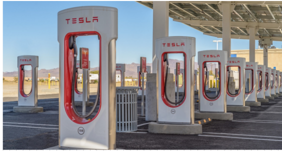
Figure 1.4: Tesla Supercharger Charging station for charging electric vehicles
