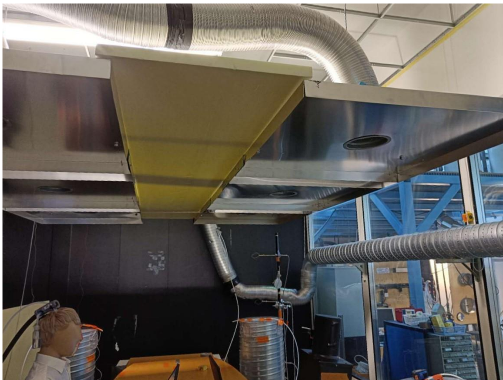
Figure 4. Perforated duct installed on the corridor side wall (simulated window in the laboratory room).
