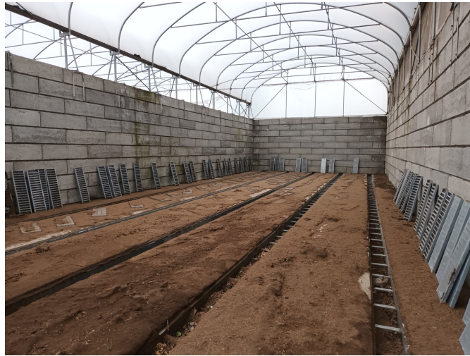
Figure 3.1: Intradel silo under study in this thesis, shown during the cleaning phase. The metal grates have been temporarily removed from the air ducts for maintenance
